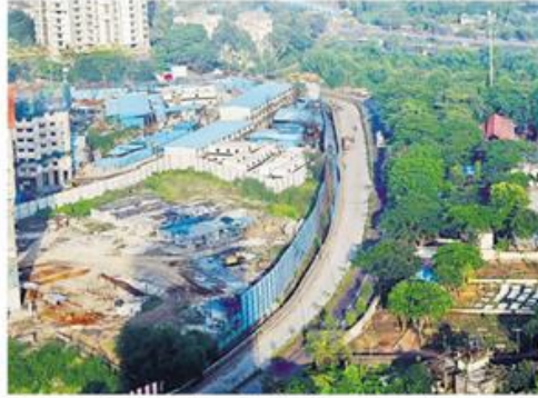
Construction for Dharavi's project-affected people near the salt pan land in Mulund East. FILE PIC/SAYYED SAMEER ABEDI
