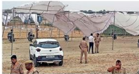
Cops keep vigil as strong winds damage the structure at the venue of Prime Minister Narendra Modi's upcoming public meeting, at Mehandiganj in Varanasi. — PTI
